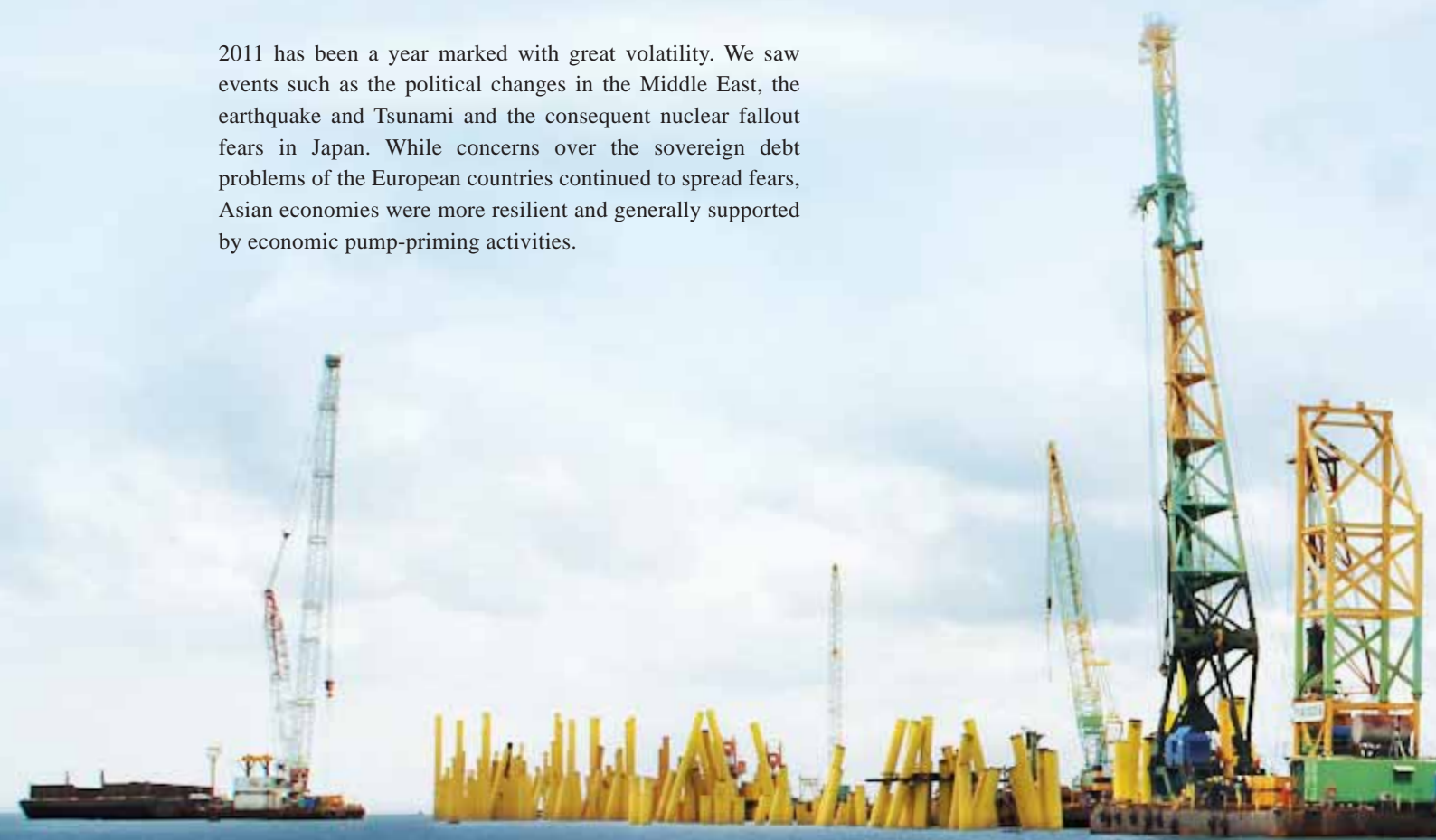
Steel pipe piles installation for LNG Regasification Project in Melaka, Malaysia for Petronas Gas Berhad
