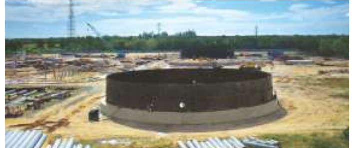
Engineering, Procurement and Construction of the Central Oil Distribution Terminal ("CODT") in Tanjung Manis, Sarawak
