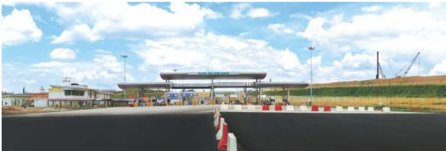
Toll Plaza construction work in progress for South Klang Valley Expressway ("SKVE") Project
