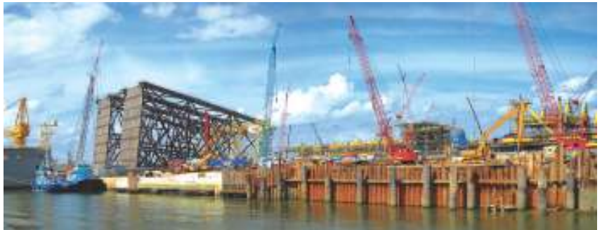
Deepwater Berth construction at MMHE, Pasir Gudang Johor for Gemusut Kakap Project
