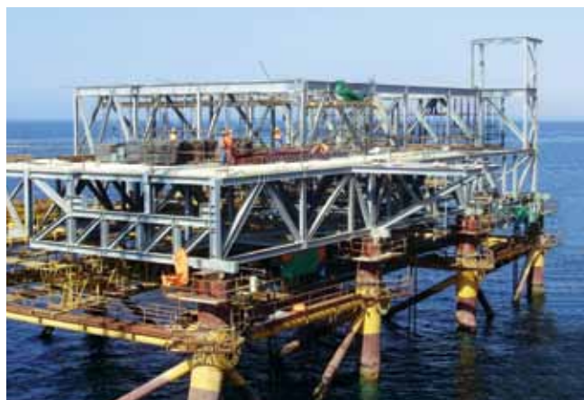
Loading Platform Jackets fabricated by Muhibbah Steel Industries Sdn Bhd for the Yemen LNG Jetty 1 Project in Balhaf, Yemen
