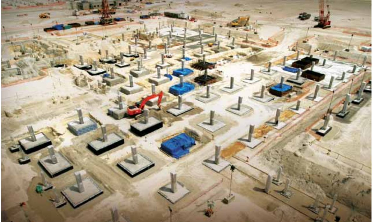
Foundation and Pile Caps for Catering Facilities Building, New Doha International Airport, Qatar
