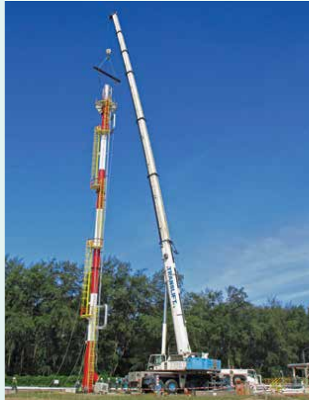
Provision of Flare System for New Ethylene Export Facility, Kerteh by Intelligent Automation Group.
