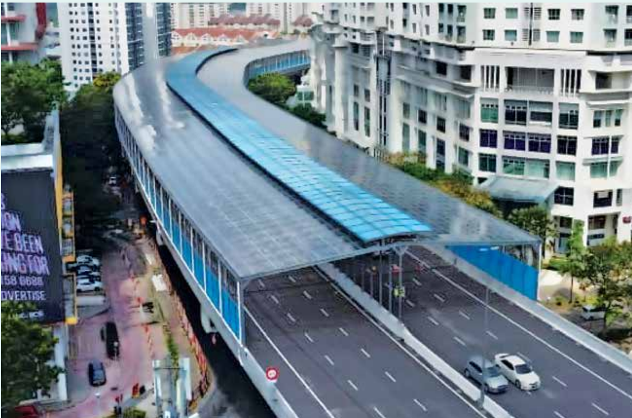
Noise Barrier for Damansara Shah Alam Highway (DASH) to reduce noise pollution
